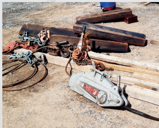
Slip on joint by tirforts
